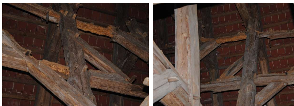
Photo 3, 4. Corroded supporting-dead bolt wall elements
