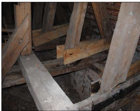
Photo 9. Corroded truss beam ends are reinforced with counter battens from boards
