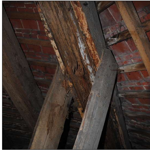
Photo 8. Corroded rafter secondary reinforced with counter battens
