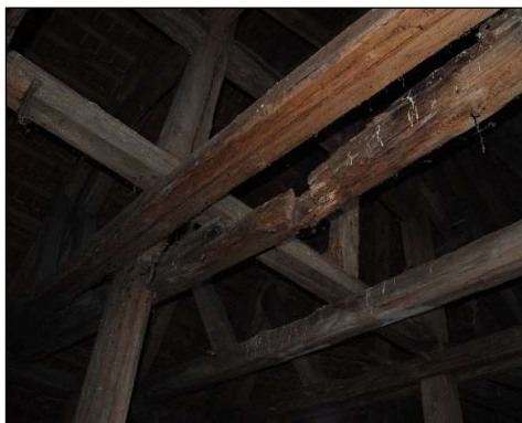
Photo 11. Place after the removed pole, biological corrosion of the collar beam
