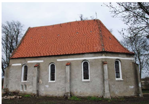
Photo 1. South view. Visible deflection of the ridge, roof slope deformation
