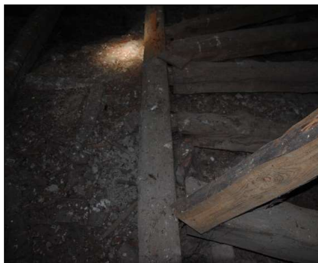
Photo 12. Split connections of truss beams above the presbytery
